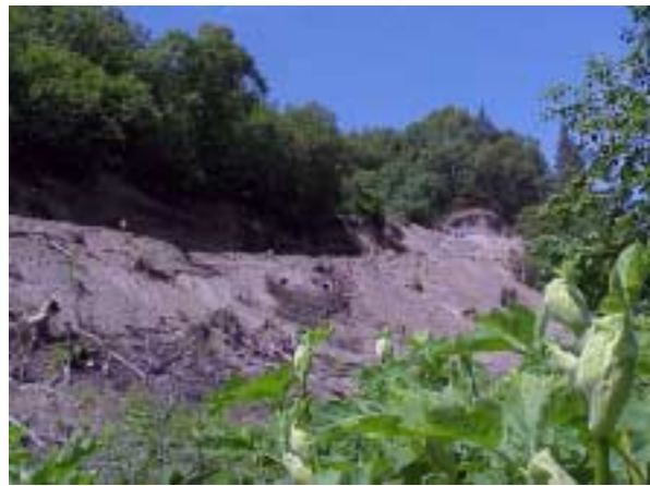
Road development taking place on steep slope above Woodard creek and monitoring site KB-180.
