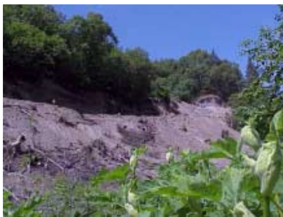
Road development taking place on steep slope above Woodard creek and monitoring site KB-180.
