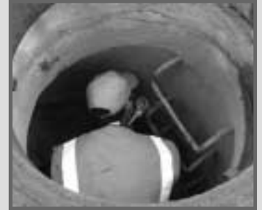
Keeper staff member, Edan Badajos, enters a man hole on Pioneer Avenue to monitor stormwater as part of the Bartlett Road Construction Project.
