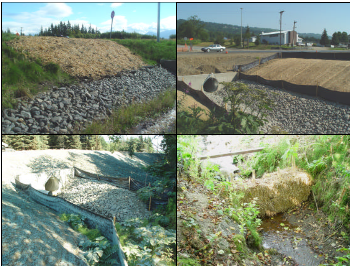
Figure 2. Examples of BMPs employed on the East End Road construction project. Upper left – straw mulching and rock-lined channel at the upstream site on Mariner Creek 9/6/05. Upper right - silt fence barriers, rolled erosion control products, and outlet protection at the downstream site on Mariner Creek 7/13/04. Lower right – straw bale barrier at the downstream site on Alder Creek 8/13/04. Lower left – seeding, silt fence barriers, and outlet protection at the downstream site on Mattox Creek 8/10/04.
