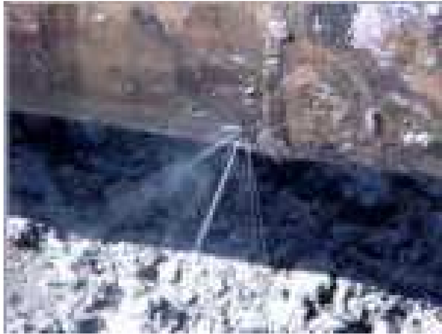
Figure 3. August 1, 2001 photo of the Tesoro 10” transmission pipeline spill in Captain Cook State Recreation Area. The pinholes spraying petroleum products (i.e., jet fuel, diesel) likely are the result of corrosion, possibly related to metal interactions with the nearby Phillips Petroleum natural gas pipeline. Photo source: Alaska Department of Environmental Conservation website.
